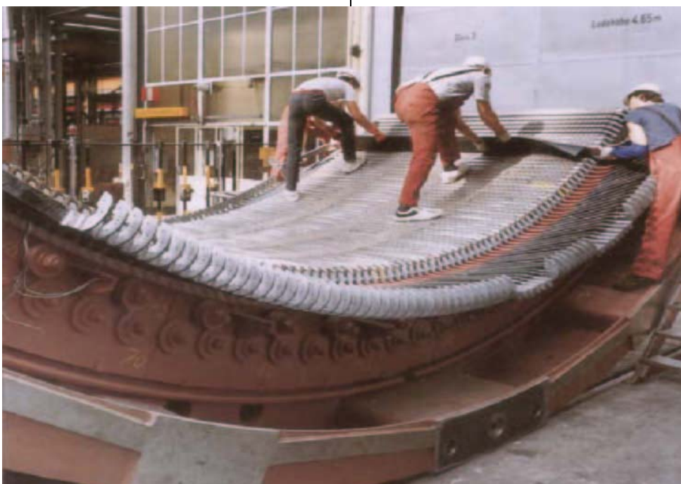
Fig.2 Inserting winding bars with a conductive slot liner and conductive resin putty
