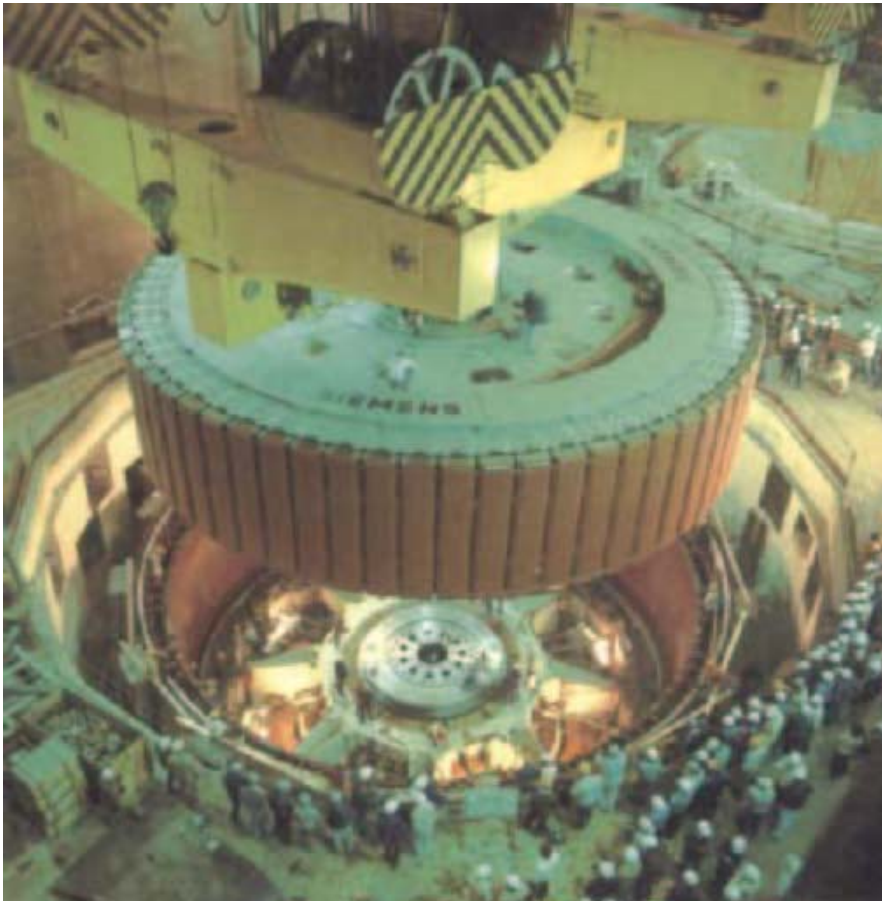
Fig. 1 Insertion of a rotor at the Itaipú hydroelectric power plant. Due to its diameter of 16 m and weight of 1960 t, assembly on site is the only practicable approach.
